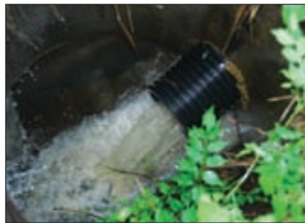
PROBLEM SOLVED: Two miles of underground pipe solved water problems on 80 acres.
